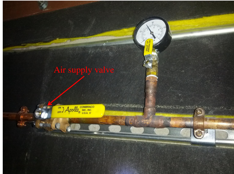
Figure A.8: Photo of a valve responsible for controlling the flow of pressurized gas from the building supply line. One valve controls flow to the room air springs, and another controls flow to the table air springs.
